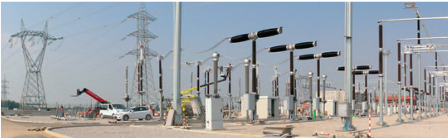
Terna Stazione 380/132 kV / Terna station 380/132 kV
